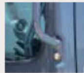
Easily repaired bolted handrails
